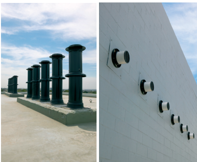
Older style roof cowls and horizontal terminals all terminating at the same height
