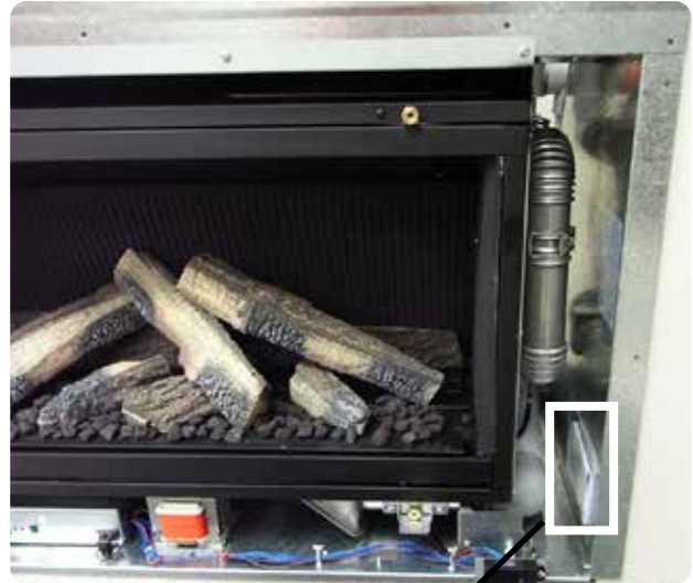
Commissioning sheet—located inside a plastic pouch inside the unit (right hand side)
