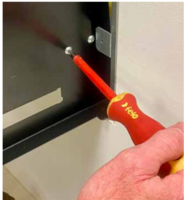
Reflector drive motor securing screws on the outside of the firebox
