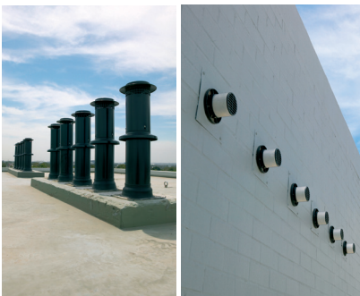
Older style roof cowls and horizontal terminals all terminating at the same height
