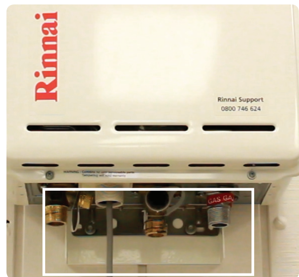
Rear security bracket installed behind water heater bracket
